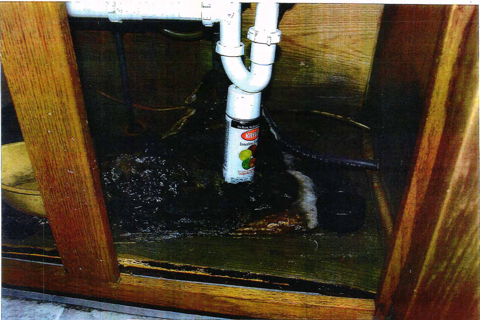
Improperly supported p-trap, unknown leakage, Ordinance Item H. Sanitary Drainage 288
